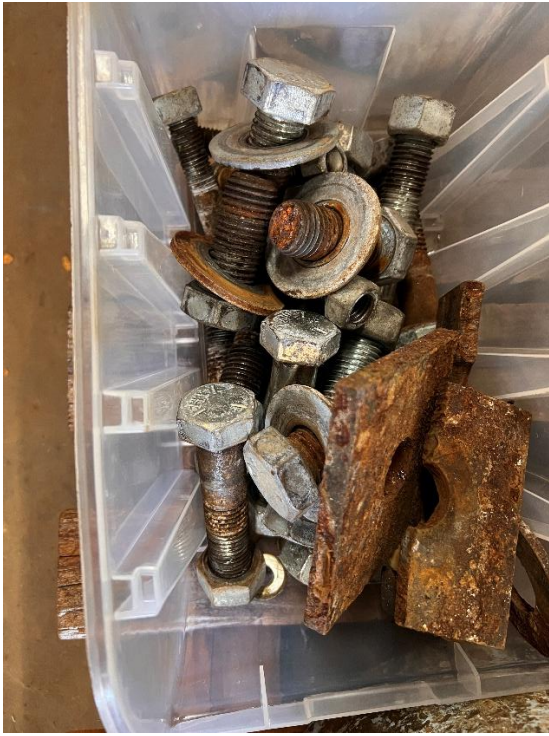
Photo #13: View of Bolts and Metal Spacers Used for the Discharge Head.
