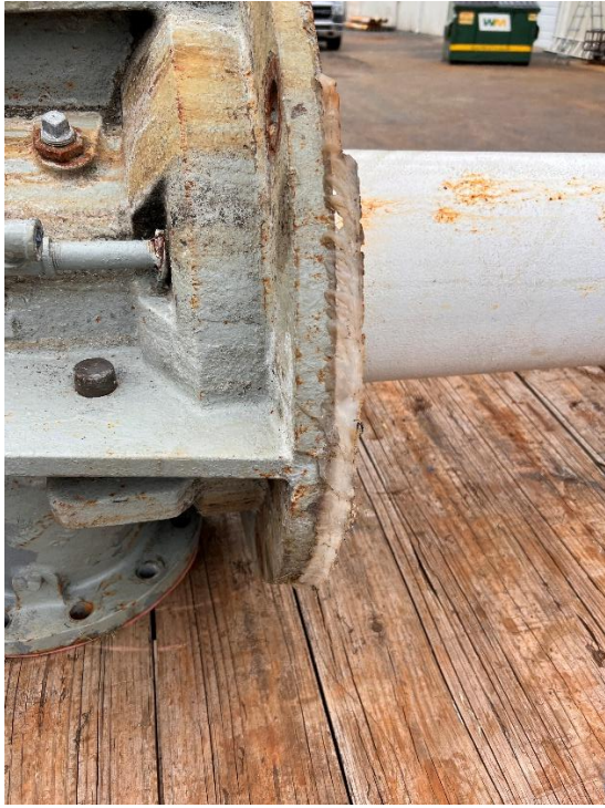
Photo #1: Discharge Head with Large Amount of Silicon Sealant. Head Had Several Large Metal Spacers Under it For Leveling Purposes.
