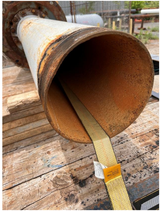
Photo #2: View of Bottom Of Discharge Head Pipe. The Threads Showed Signs of Being Dropped Before Installation. The Bent Threads Allowed A Leak To Form.
