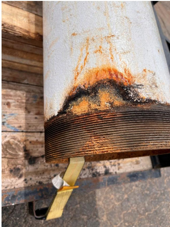
Photo #3: Close-up of the Discharge Head Pipe. Signs of Water Leaking by the Threads is Visible. The Threads in This Area of the Pipe Show Signs of Heavy Corrosion.
