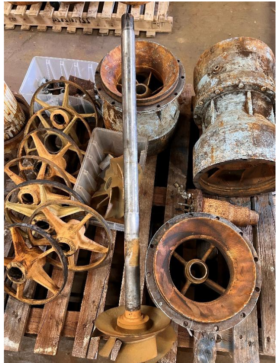
Photo #12: View of Pump Bowls, Impellers, Pump Shaft, Spider Bearings, Stuffing Box and Miscellaneous Bolts.
