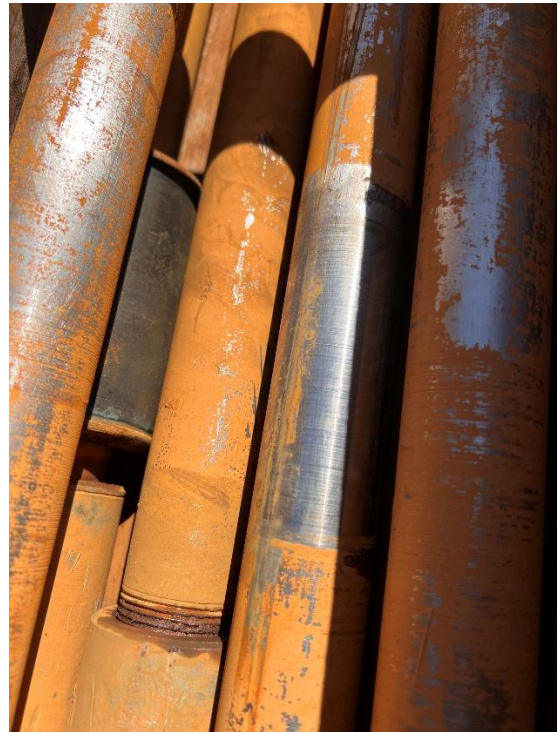
Photo #8: View of Line Shafts. Moderate Wearing Can Be Seen Where The Spider Bearing Bushings Sit on the Shaft
