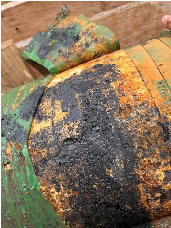
Photo #7: Close-up View of Pitting Under the Tape.
