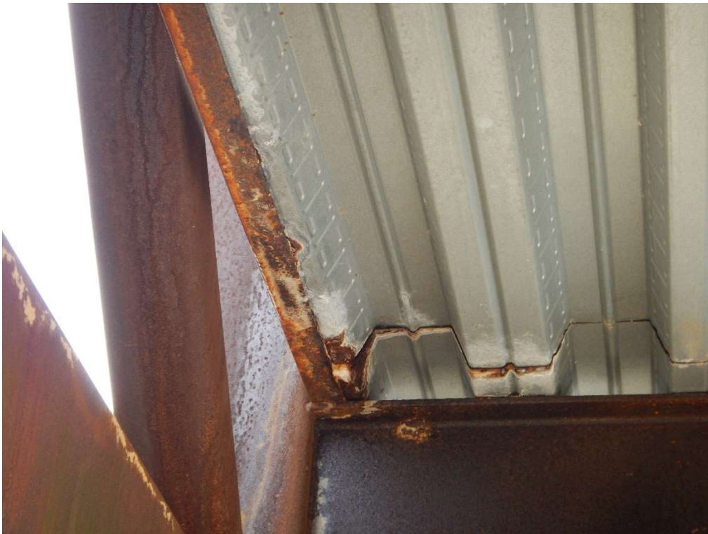
Stay-in-Place Form Edge Deterioration
