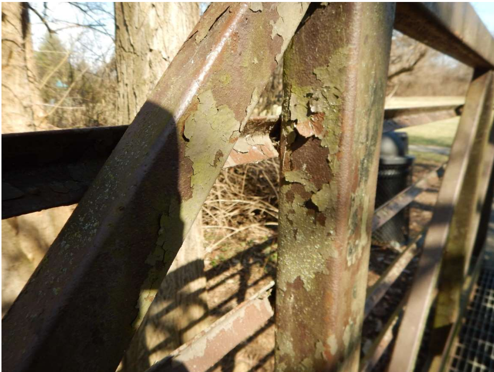
Typical Flaking Paint
