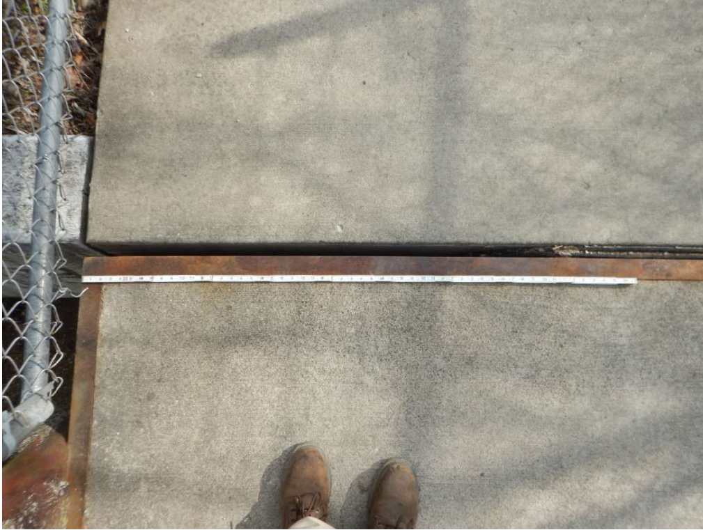
Failing Deck Joint, South End of Bridge
