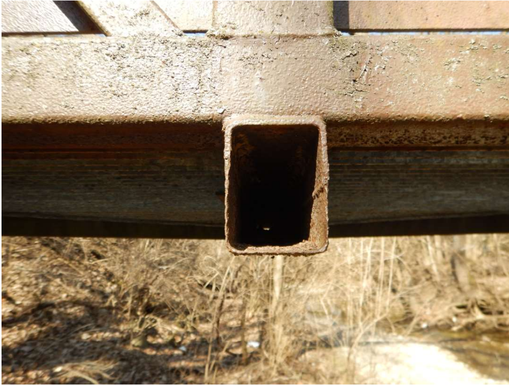
Floor Beam Deterioration
