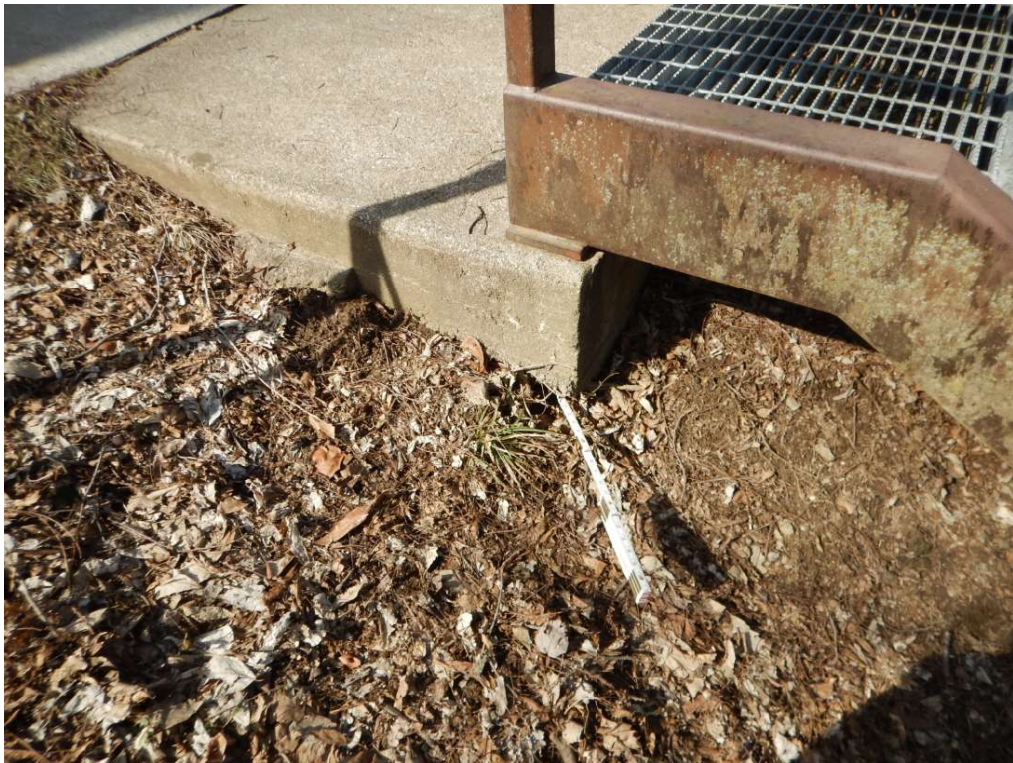
Undermining at Stairway Pad
