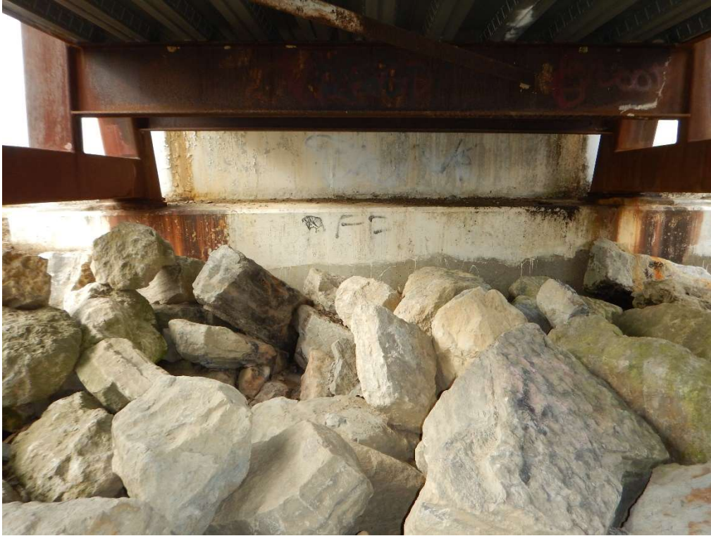
Abutment Staining, North End of Bridge
