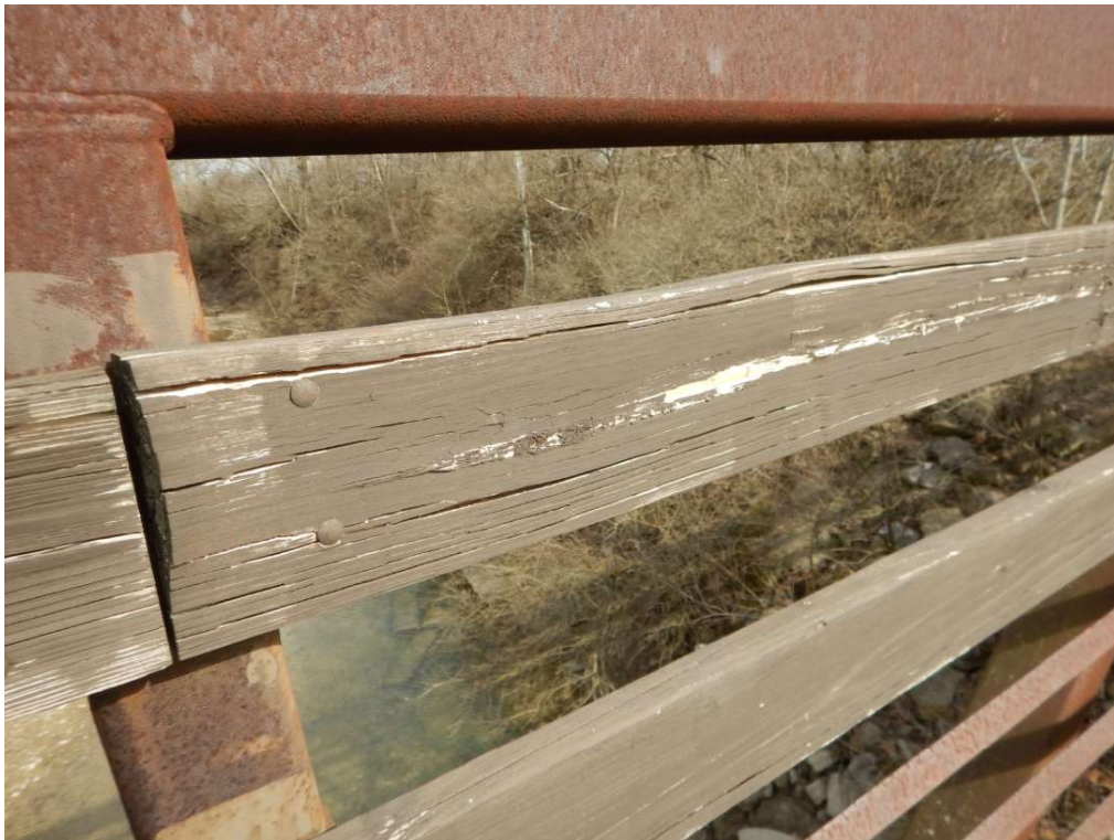
Timber Railing Deterioration
