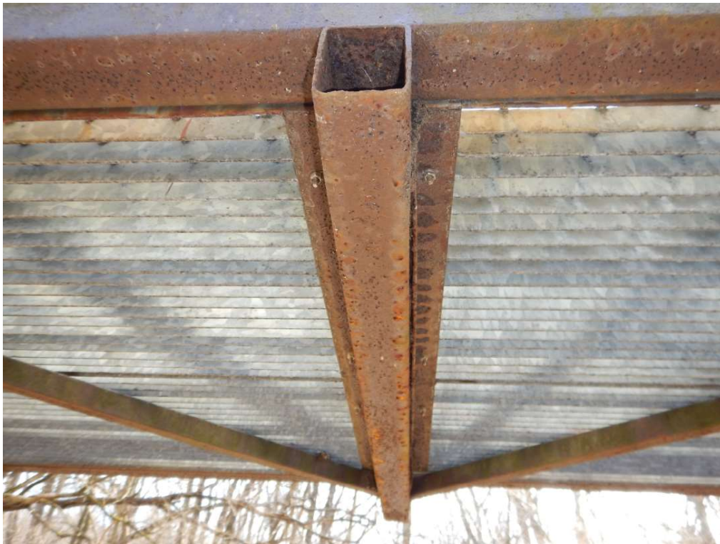
Floor Beam Deterioration
