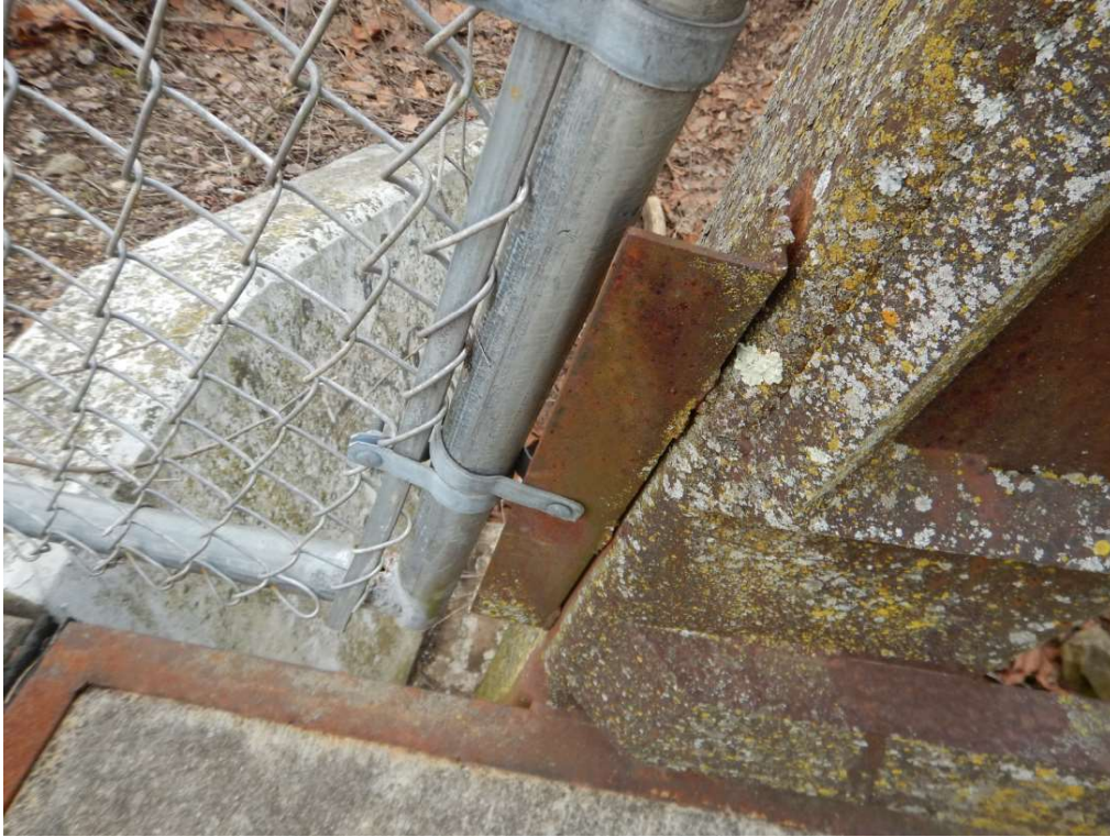
Broken Approach Fence Weld Connection
