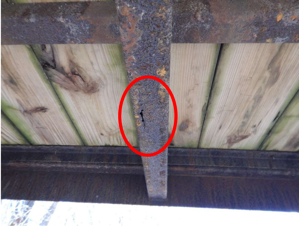
Perforation in Floor Beam 5
