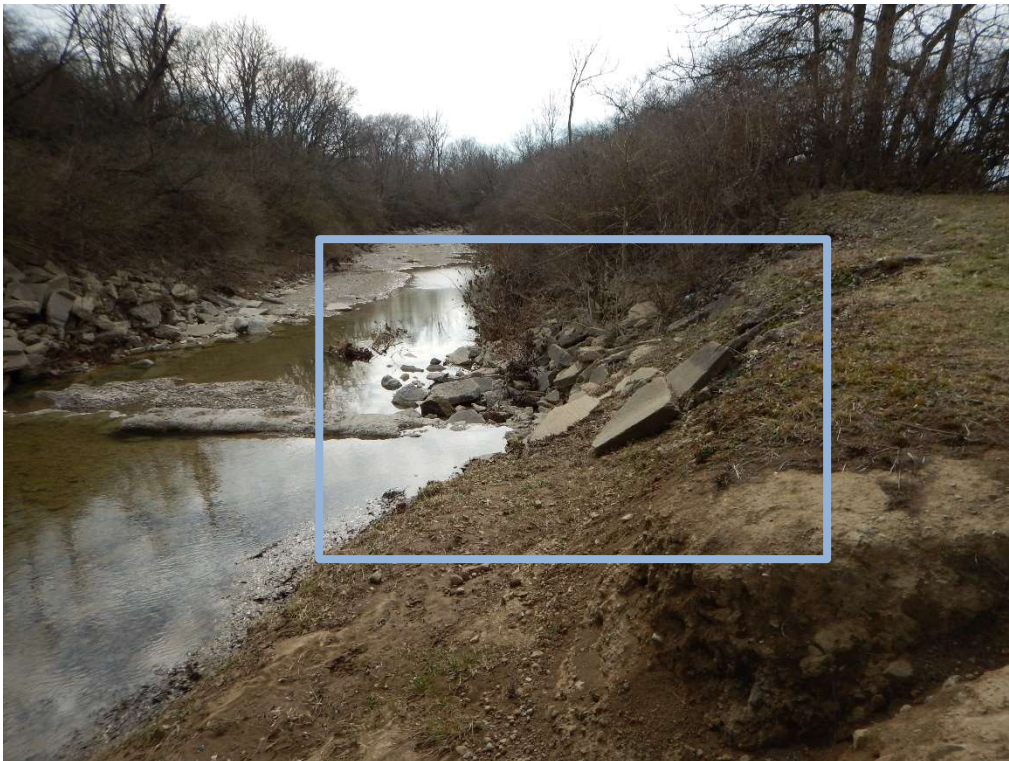
Erosion Along North Embankment (Note: Rock Channel Protection Washing Out)
