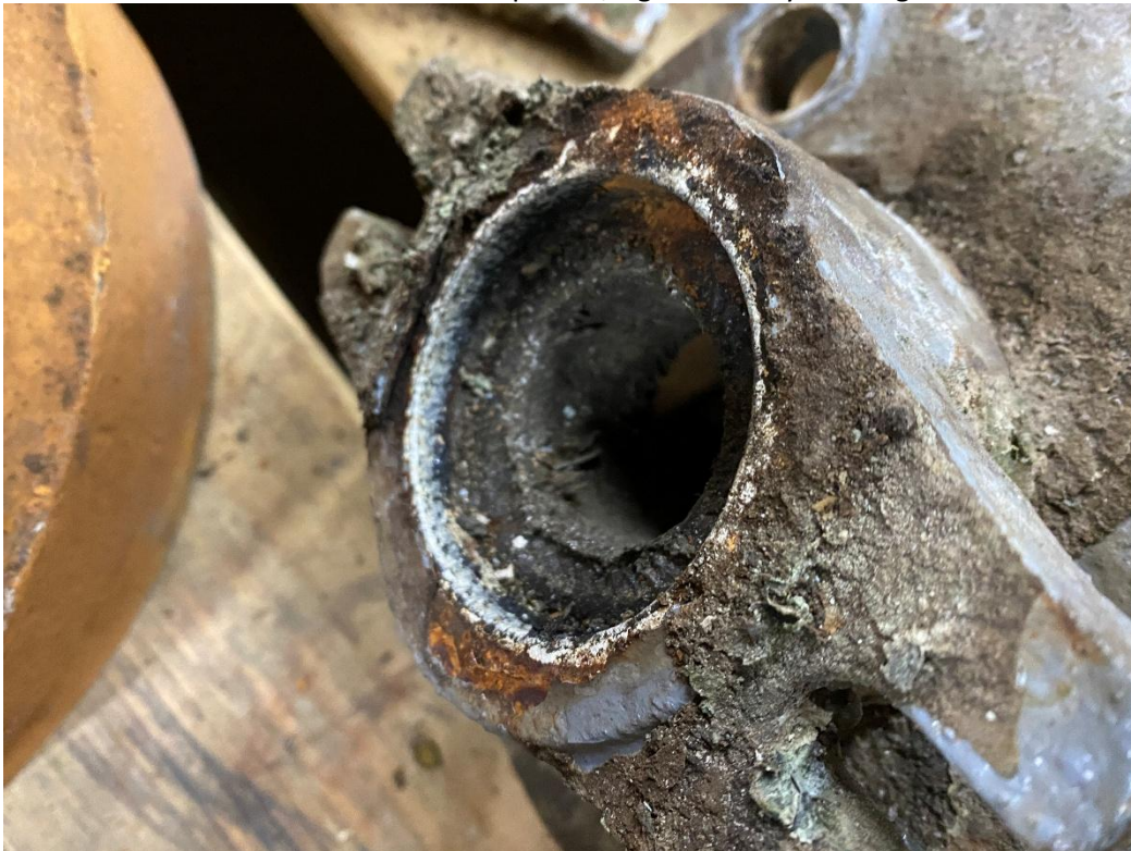
Photo 4: View of Stuffing Box and Packing Gland
