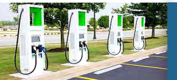
Electric vehicle charging stations
