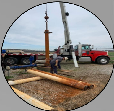
Owner's Pump Removed
