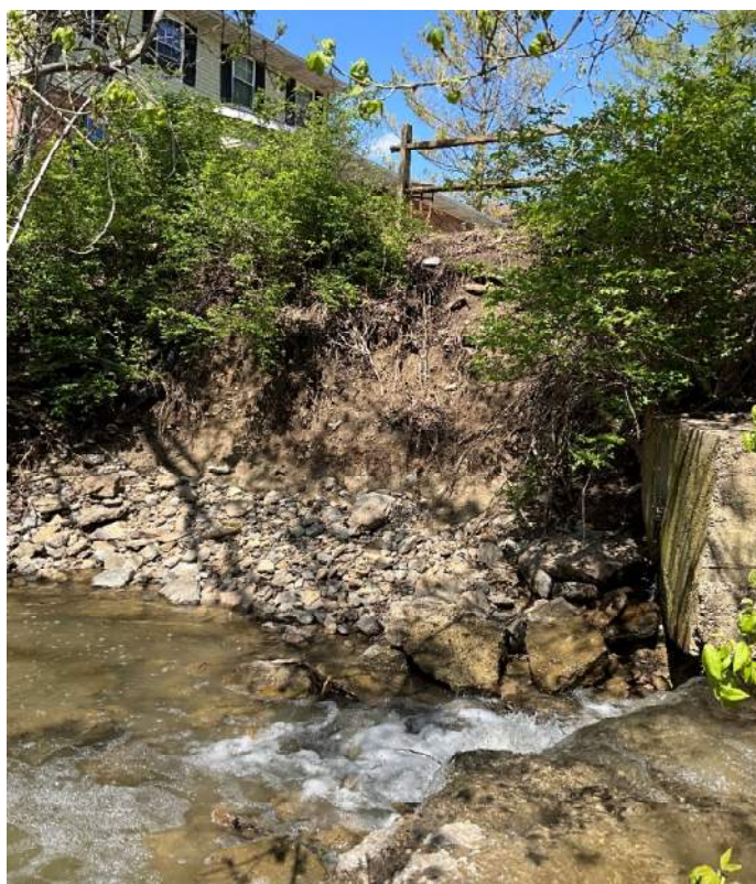
Photo 12 – Northwest Embankment Erosion
