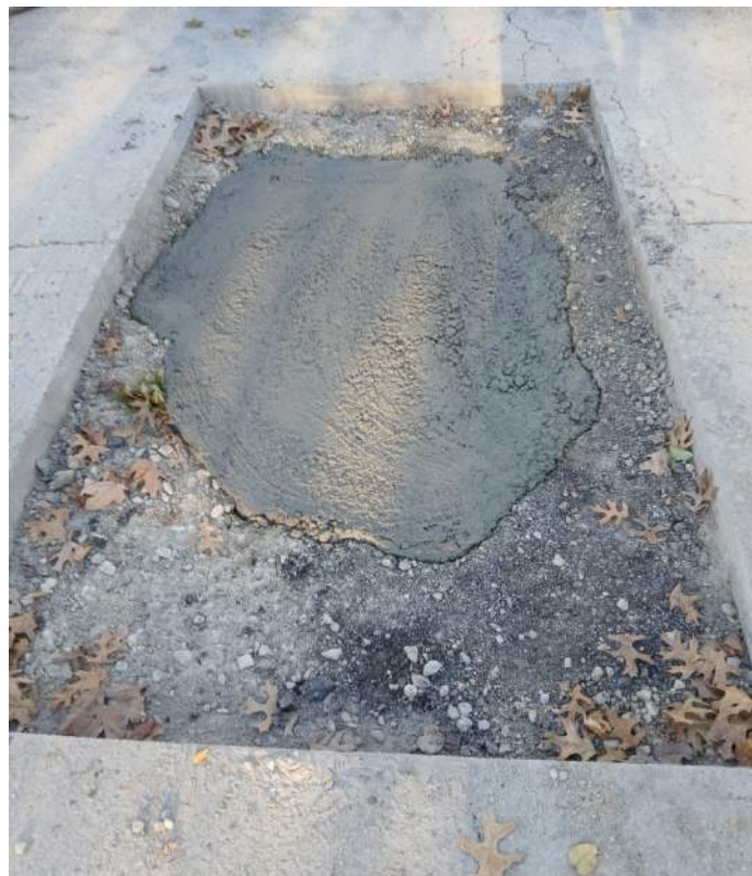
Photo 10 – Patch of Void Beneath Roadway Due to Material Loss through Existing Arch Walls (2024)
