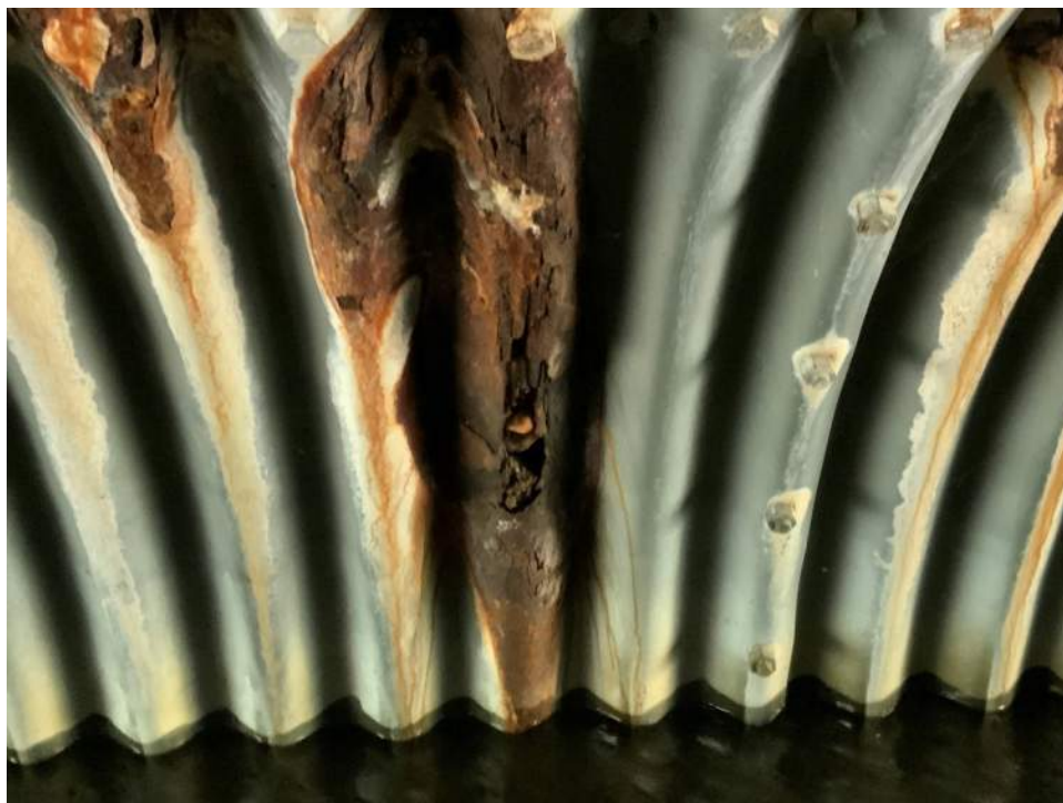
Photo 7 – Typical Corrosion Along Bolt Lines
