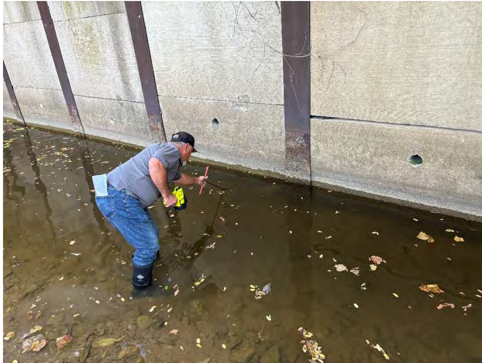
Photograph 5: Probing below bottom panel, Erosion extends about 2 feet below panel at this location.
