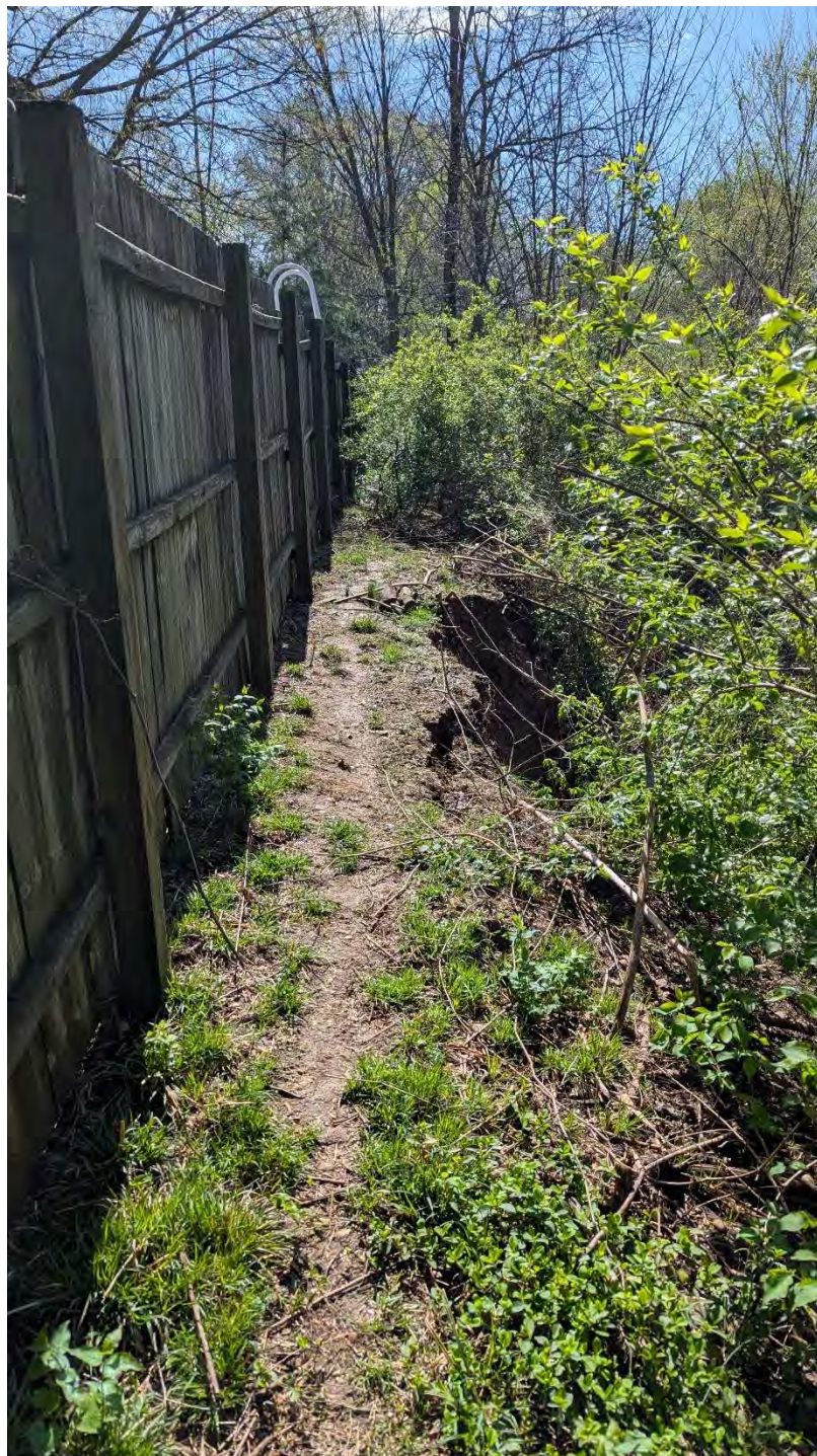
Photograph 9: Soil loss behind pier wall within rear of property at 5121 Southview Drive
