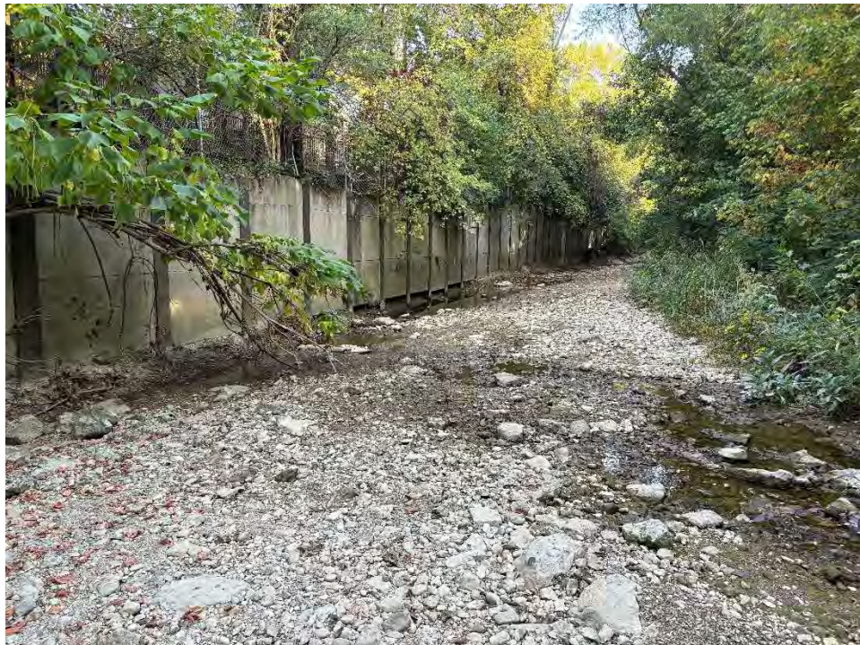
Photograph 8: Similar erosion issue occurring downslope of the subject area.
