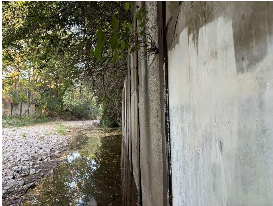
Photograph 6: Top of pier wall visibly rotating.
