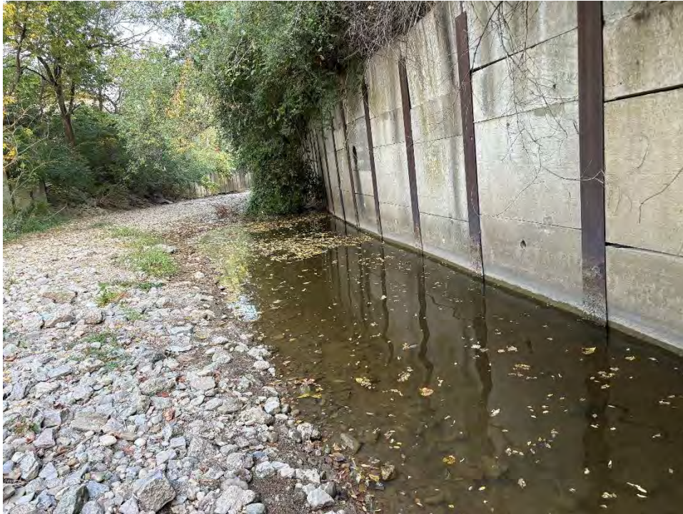
Photograph 1: View of eroded area in front of pier wall.
