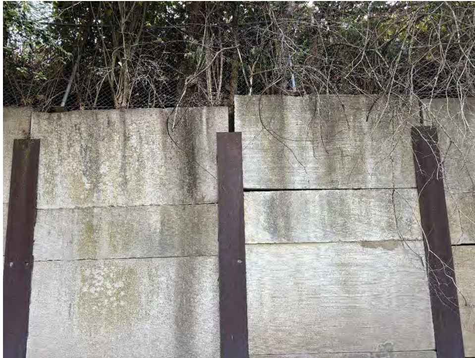
Photograph 7: Differential panel movement
