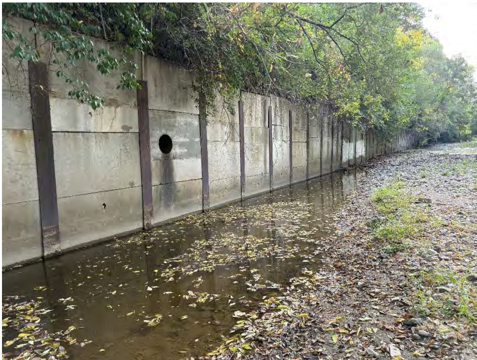
Photograph 2: View of eroded area in front of pier wall.
